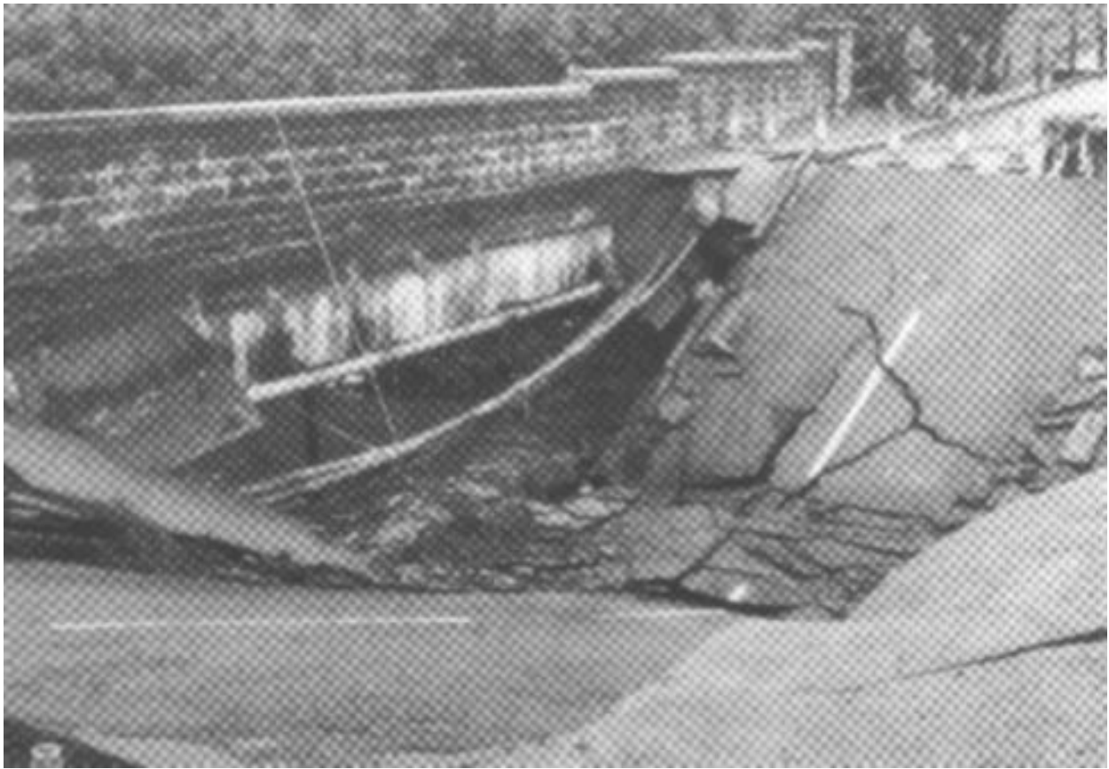
Fig 1.20 - Trop tard.... [tiré de Pritchard B. 1992 Bridge design for economy and durability , Thomas Telford Services London, 172 p.]
